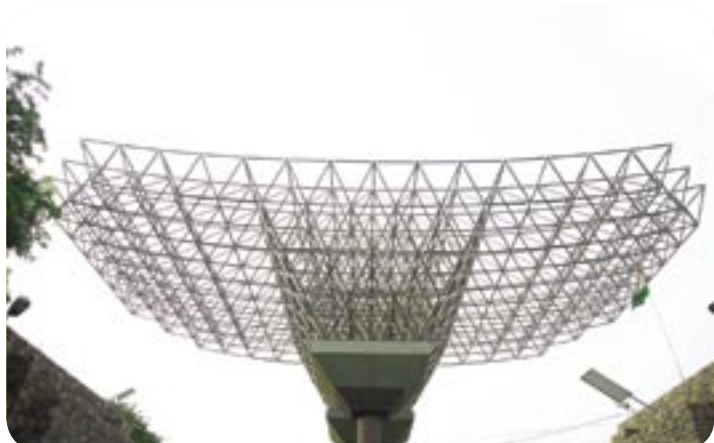
Stainless Steel Space Frame at the Entrance of Hisar Plant
