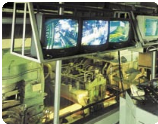
The Control Room of the Hot Steckel Mill
