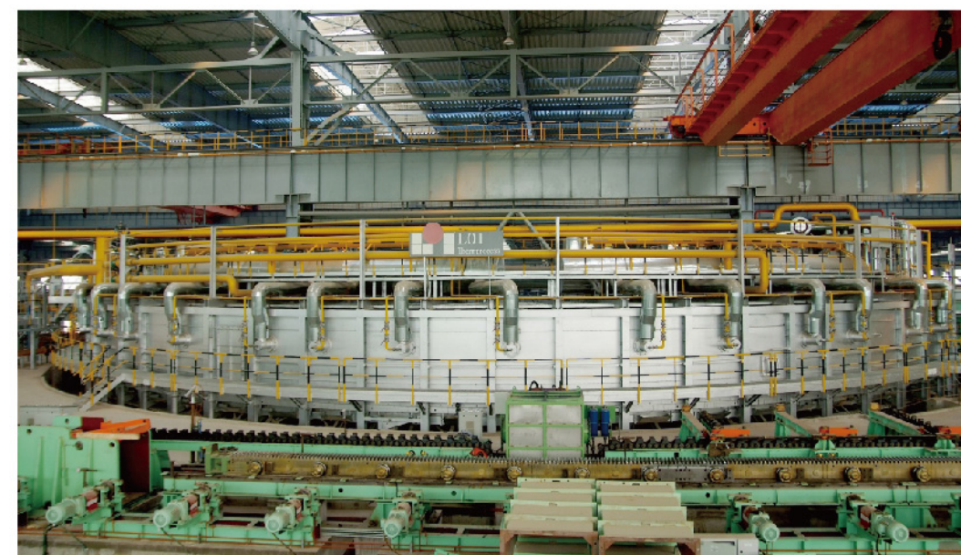
● 环形加热炉 Ring shape furnace
