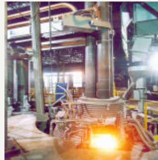
STEEL REFINING LADLE FURNACE
